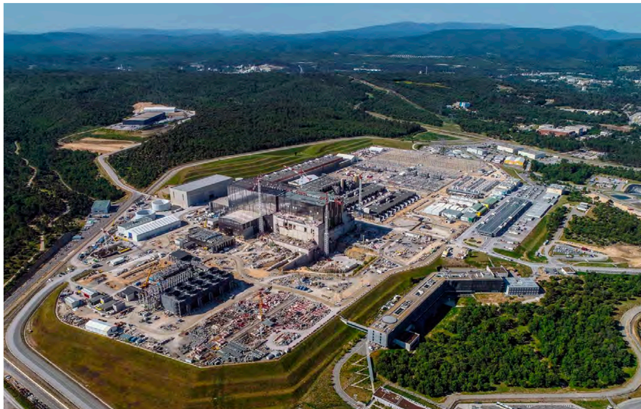
Fot. 6. Obszar budowy reaktora ITER, stan na 27 maja 2020. (fot. ITER Organization, EJF Riche) Photo 6. The ITER reactor construction area, as of May 27, 2020 (Photo: ITER Organization, EJF Riche)
