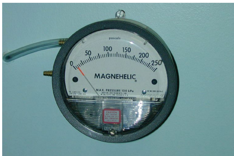
Figure 5.13. A Magnehelic pressure gauge, which shows that air pressure in the room is slightly higher than that in the corridor
