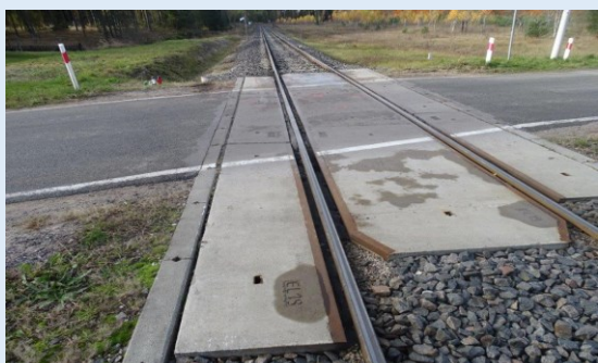
Photograph 13 - A view of the technical condition of the level crossing from the direction of passenger car's travel (source: materials provided by the railway commission)
