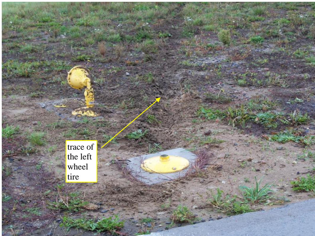
Photo 8. Damaged runway end light and trace of the left wheel of the main landing gear near THR 26.
